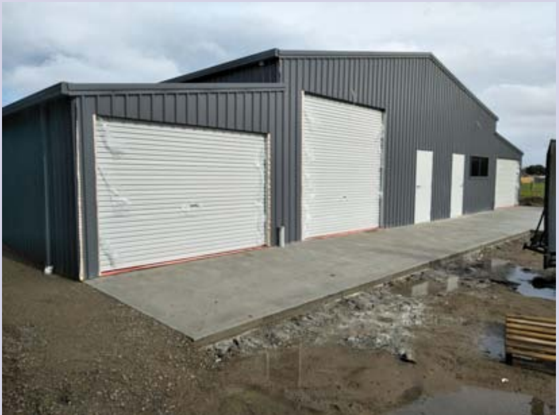
Since this photo was taken, the apron in front of the workshop has been completed.
